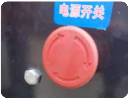
Emergency stop switch
